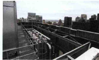
The chilled water/central plant thermal storage system on the rooftop of TIAA-CREF's headquarters building in Manhattan.
