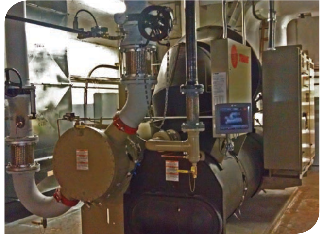
A 290-ton centrifugal chiller with a variable frequency drive provides energy savings and enhances resident comfort.
