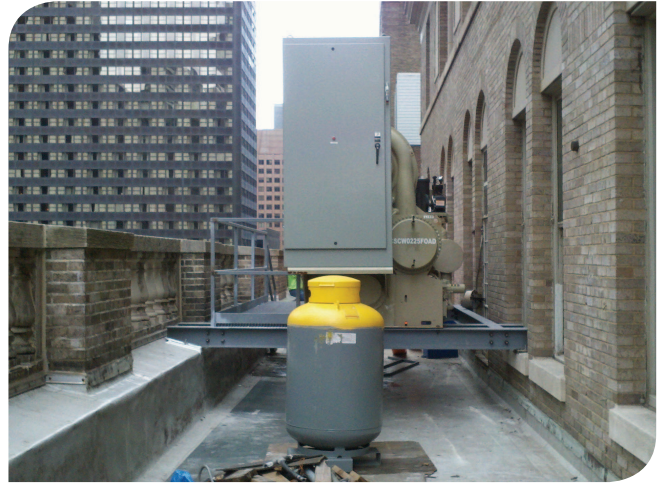
Trane built a steel structure to balance the equipment's weight between the parapet and a windowsill.
