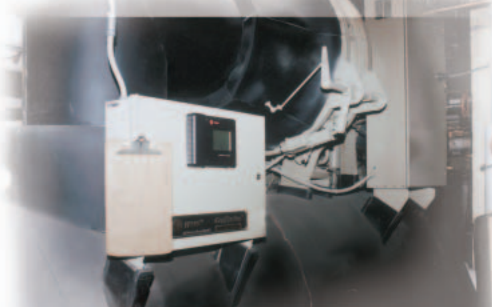
Because of tight clearances, the chillers were moved into the building in sections and assembled in place.
