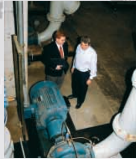
Constant speed chilled water pumps optimize efficiency of the plant.
